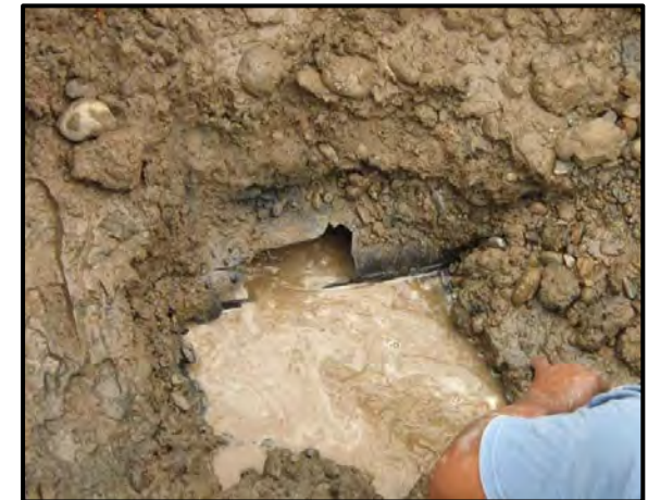
Break FOFO pipe
