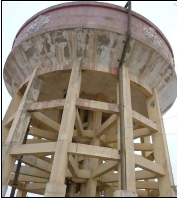
Storage Tank Damage
